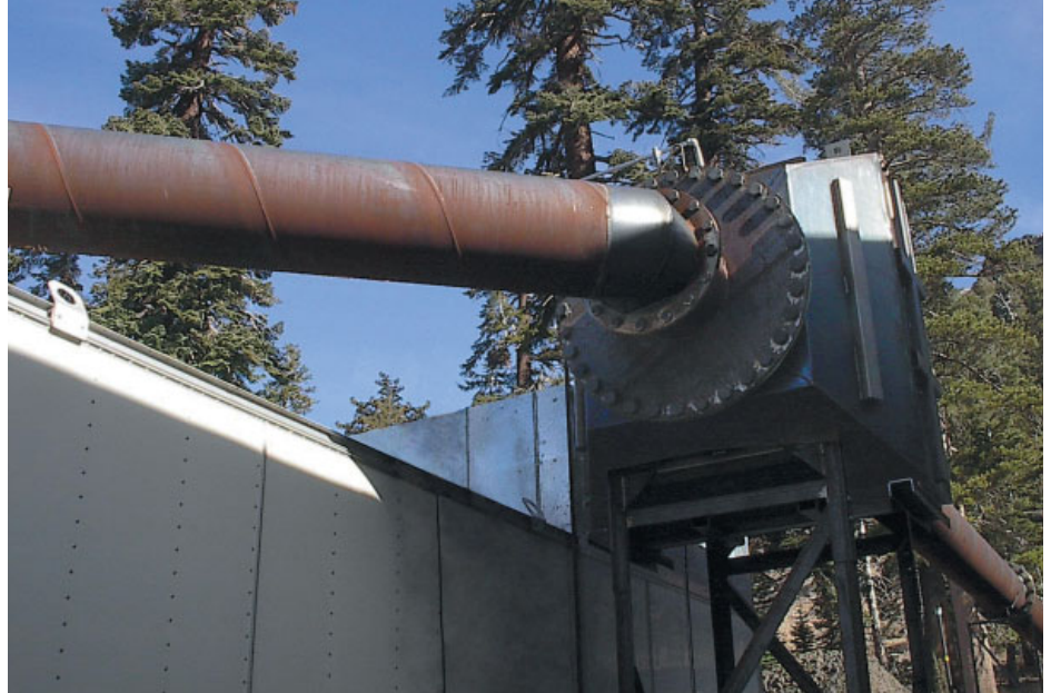
This CombiKat® diesel particulate filter is reducing to some of the nation's lowest regulatory limits exhaust particulates from a brand new Cat 3516C diesel engine installed in a prime power application at Mountain Utilities in Kirkwood, Calif.
